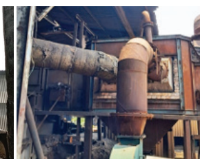
Recuperator system installed
