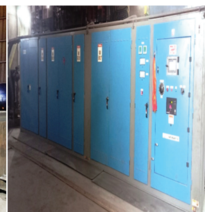
New EE induction furnace
