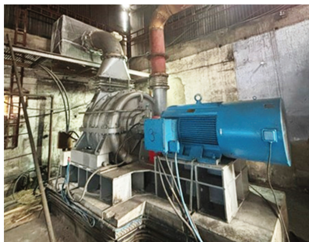
New EE centrifugal blower
